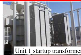
Unit 1 startup transformer
