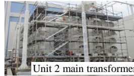
Unit 2 main transformer
