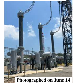
GIS in Naka Noto Sub-station
